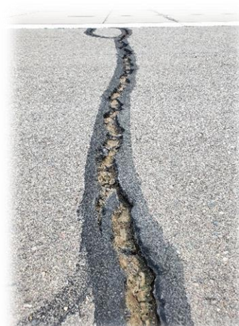
Photo 6 – Large Crack in RW Shoulder Pavement
