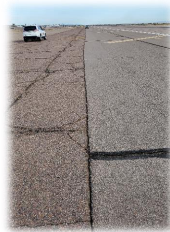
Photo 5 – Interface of RW Shoulder Pavement and deteriorated AC
