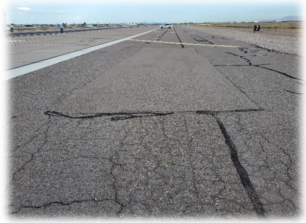
Photo 4 – Deteriorated RW Shoulder Pavement (East Side of RW)
