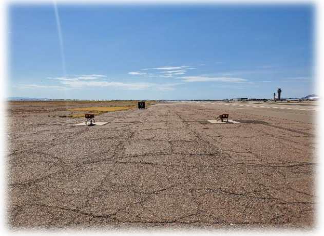
Photo 16 – RW '12R' PAPIs in Deteriorated AC Pavement
