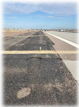
Photo 2 – RW Shoulder Pavement North of TW 'L' (West Side of RW)
