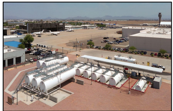
Gateway Airport's Aviation Fuel Farm
